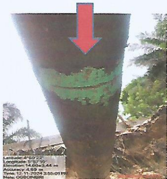
Pic1: Showing hacksaw cut on the pipeline
